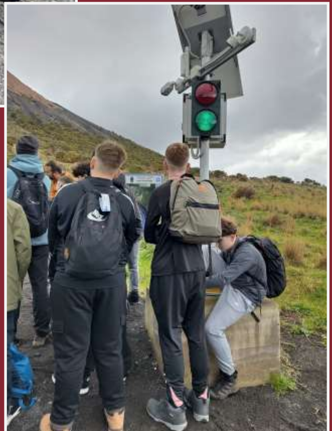
Gas measuring station at the base of Vulcano.
